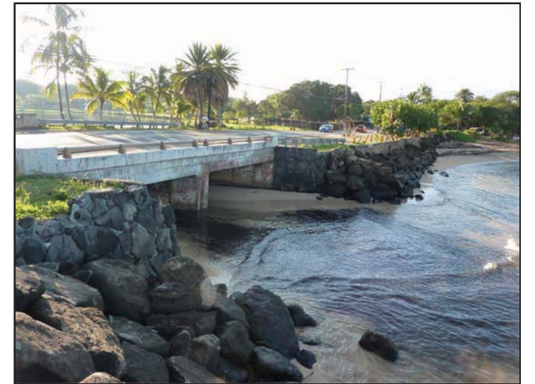
Photo 2. December 14, 2009 looking at the stream mouth from the east side of the bridge.
