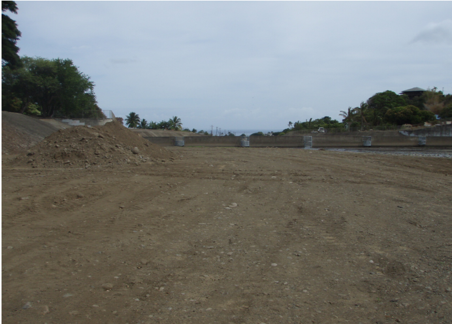
Inspect ID: ISIL_2009_a_0004 Name: Flood Reduction Chnl Caption: Sta. 130+90, Left of centerline Continue to remove stockpile of debris Unresolved
