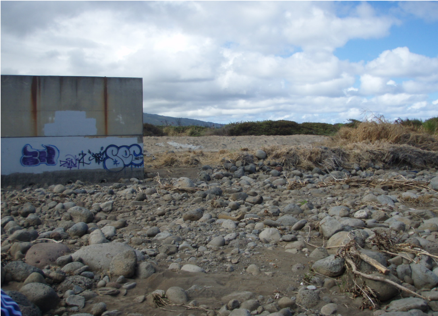
Inspect ID: ISAL_2009_a_0001 Name: Levee Embankment Caption: Sta. 4+70, LB Riprap in good condition, concrete surface in good shape
