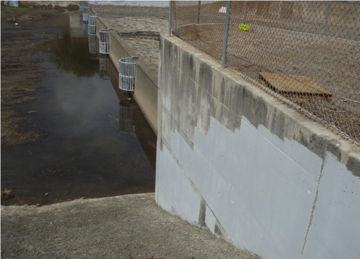
Inspect ID: ISIR_2009_a_0004 Name: Floodwall Caption: Sta. 127+20, RB No spalling, no deterioration noted
