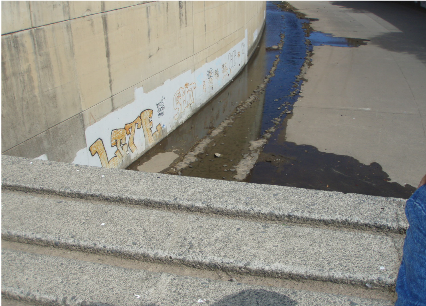
Inspect ID: ISHR_2009_a_0010 Name: Flood Reduction Channel Caption: Sta. 97+10, Centerline Concrete channel in good condition no debris no obstructions adjacent to 25 ft drop)
