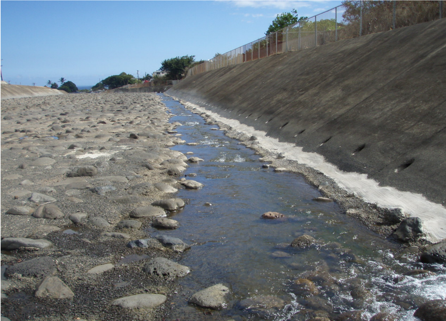
Inspect ID: ISHR_2009_a_0005 Name: Flood Reduction Channel Caption: Sta. 114+40, RB Drop Structure # 2, Sideslope repaired
