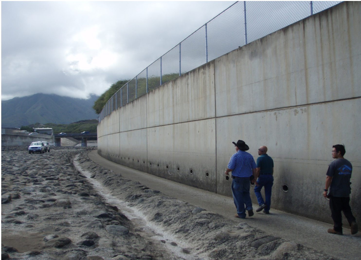
Inspect ID: ISAL_2009_a_0002 Name: Floodwall Caption: Sta. 13+70, LB Concrete floodwall in good condition, joints caulked, flapgate lubricated, fence recently replaced, weep holes clean
