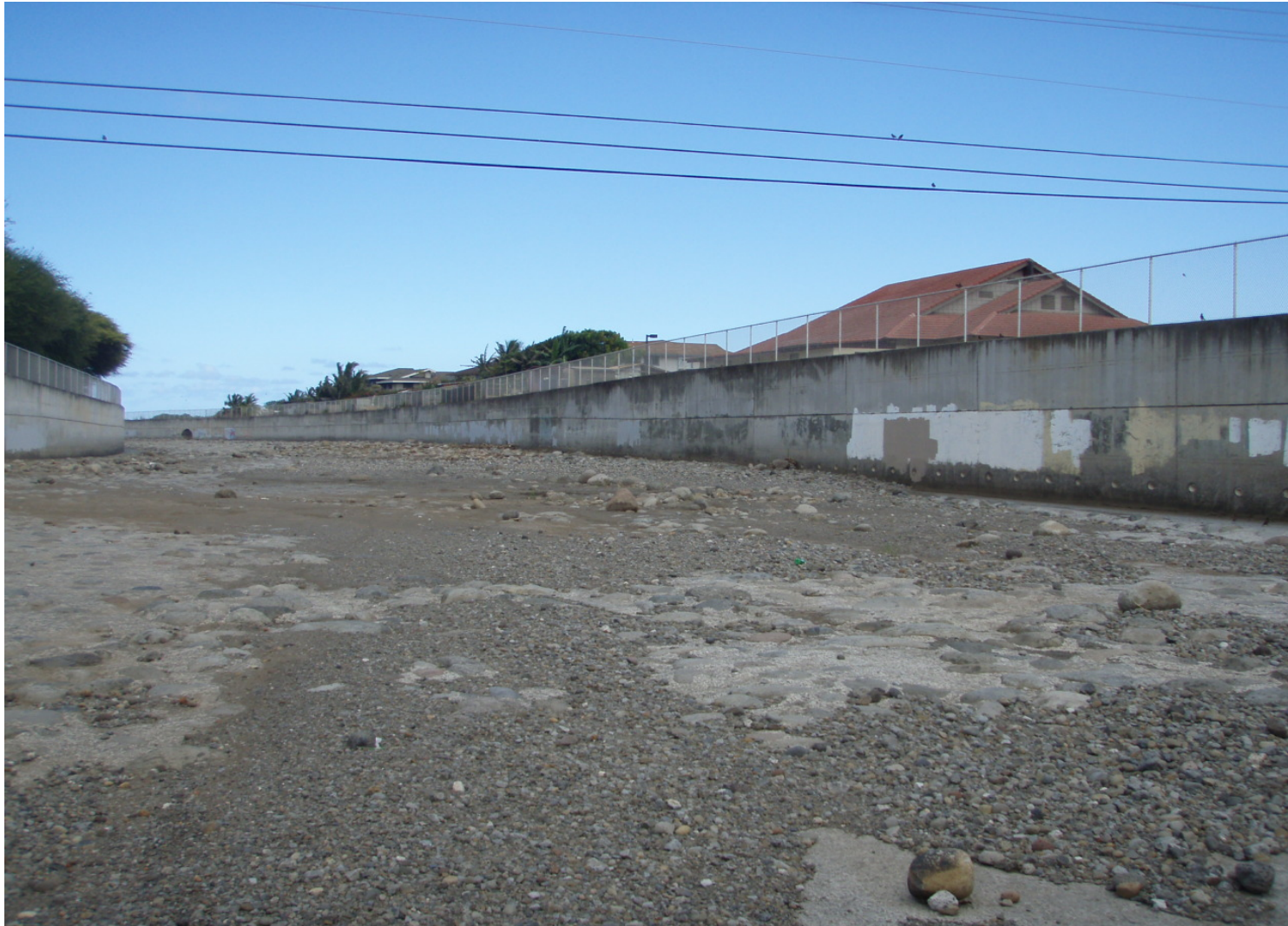
Inspect ID: ISAR_2009_a_0001 Name: Flood Reduction Channel Caption: Sta. 19+20 No major vegetation or debris in the floodway
