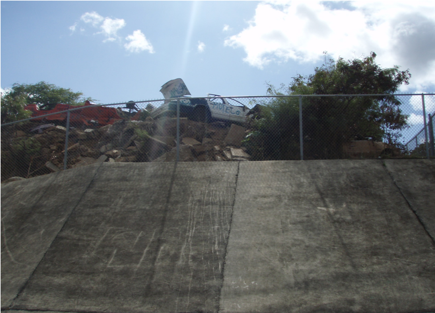
Inspect ID: ISHR_2009_a_0006 Name: Levee Embankment Caption: Sta.110+10, RB Encroachment at levee crown, Minimally Acceptable, at Drop structure # 3
