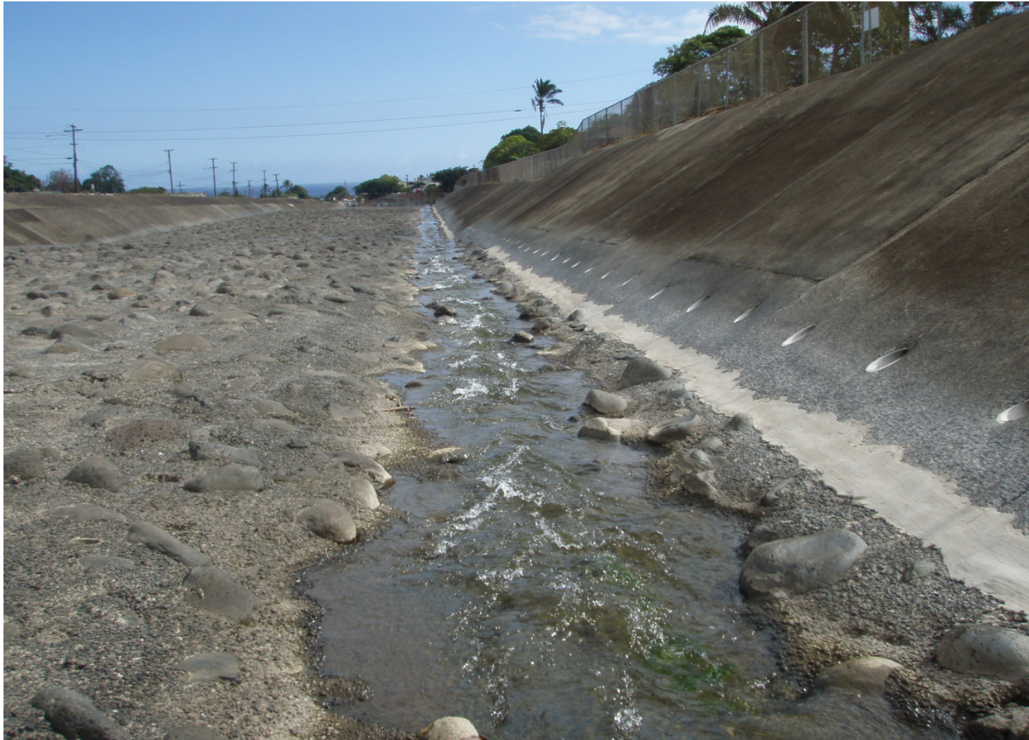
Inspect ID: ISHR_2009_a_0002 Name: Flood Reduction Channel Caption: Sta. 120+80, RB Start of recent repairs to toe/invert at low flow channel
