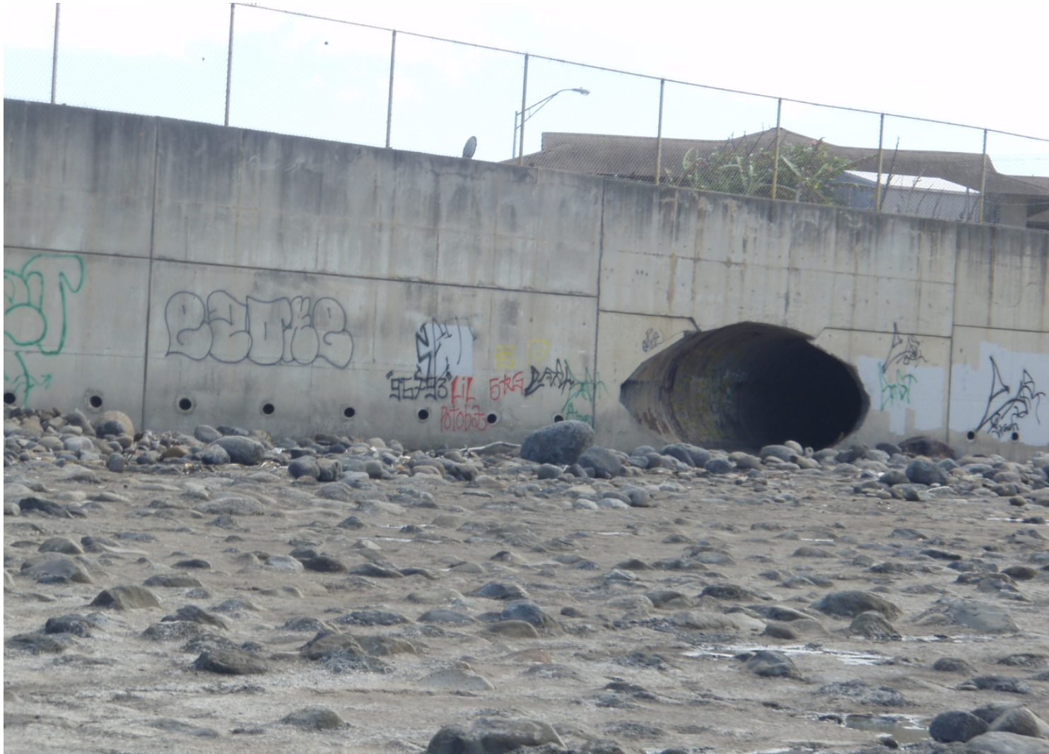
Inspect ID: ISAR_2009_a_0003 Name: Interior Drainage Caption: Sta. 6+70,RB 8 foot culvert, clear of debris and trash
