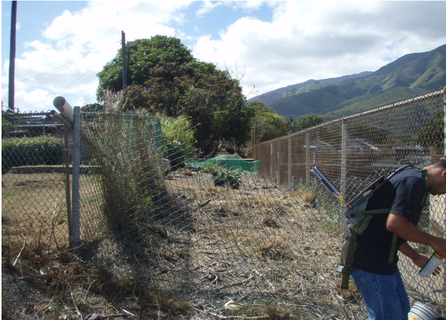
Inspect ID: ISHR_2009_a_0011 Name: Flood Reduction Channel Caption: Sta. 93+60, RB Maintenance access restblished, in good condition
