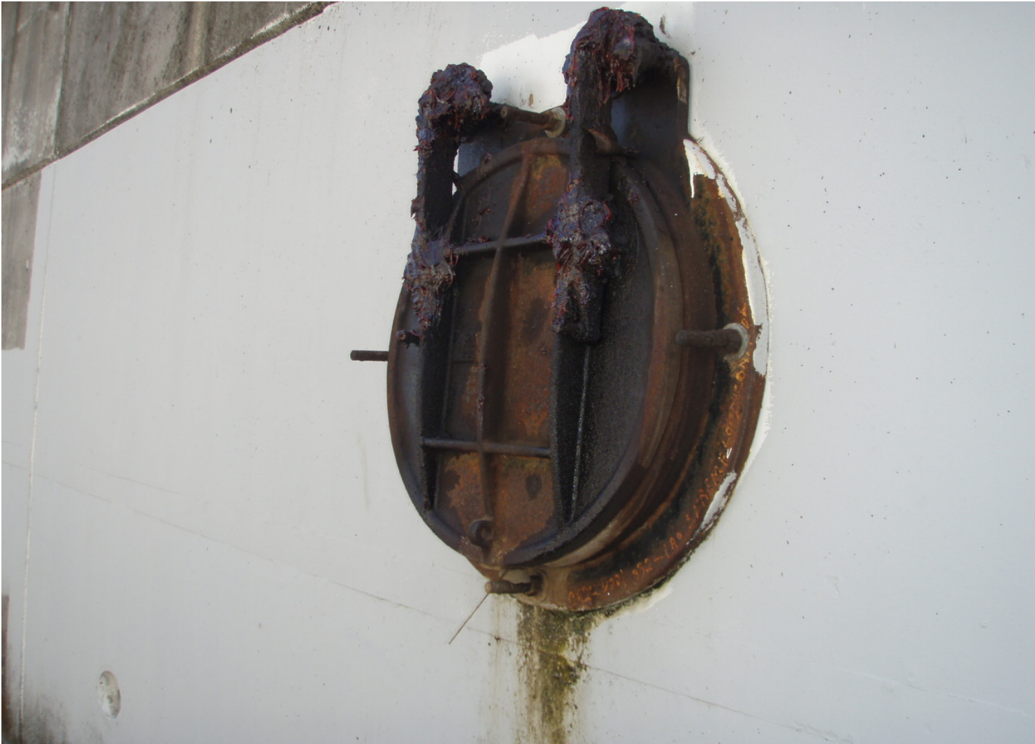
Inspect ID: ISHR_2009_a_0009 Name: Interior Drainage Caption: Sta. 97+20, RB 24 inch flapgat in good condition and greased
