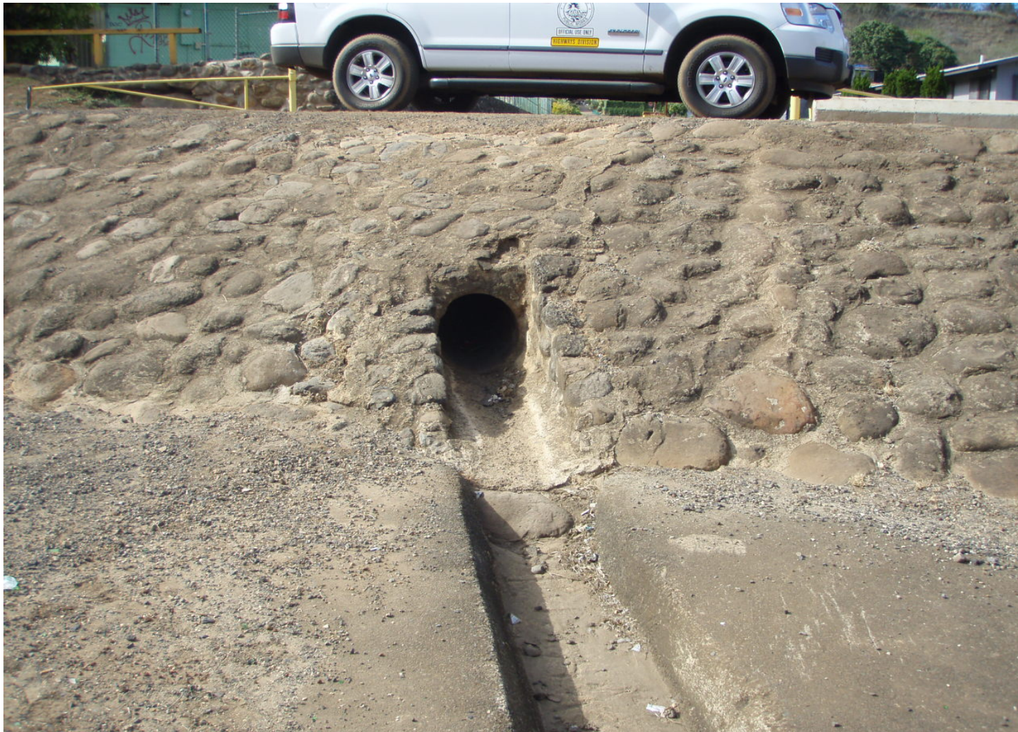
Inspect ID: ISHL_2009_a_0002 Name: Interior Drainage Caption: Sta. 118+60, LB Culvert is clear, no obstructions to flow
