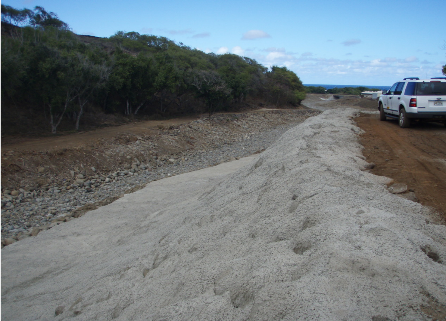
Inspect ID: ISLE_2009_a_0005 Name: Levee Embankment Caption: Sta. 40+40, (Levee B) Repair made to sideslope. Excellent work
