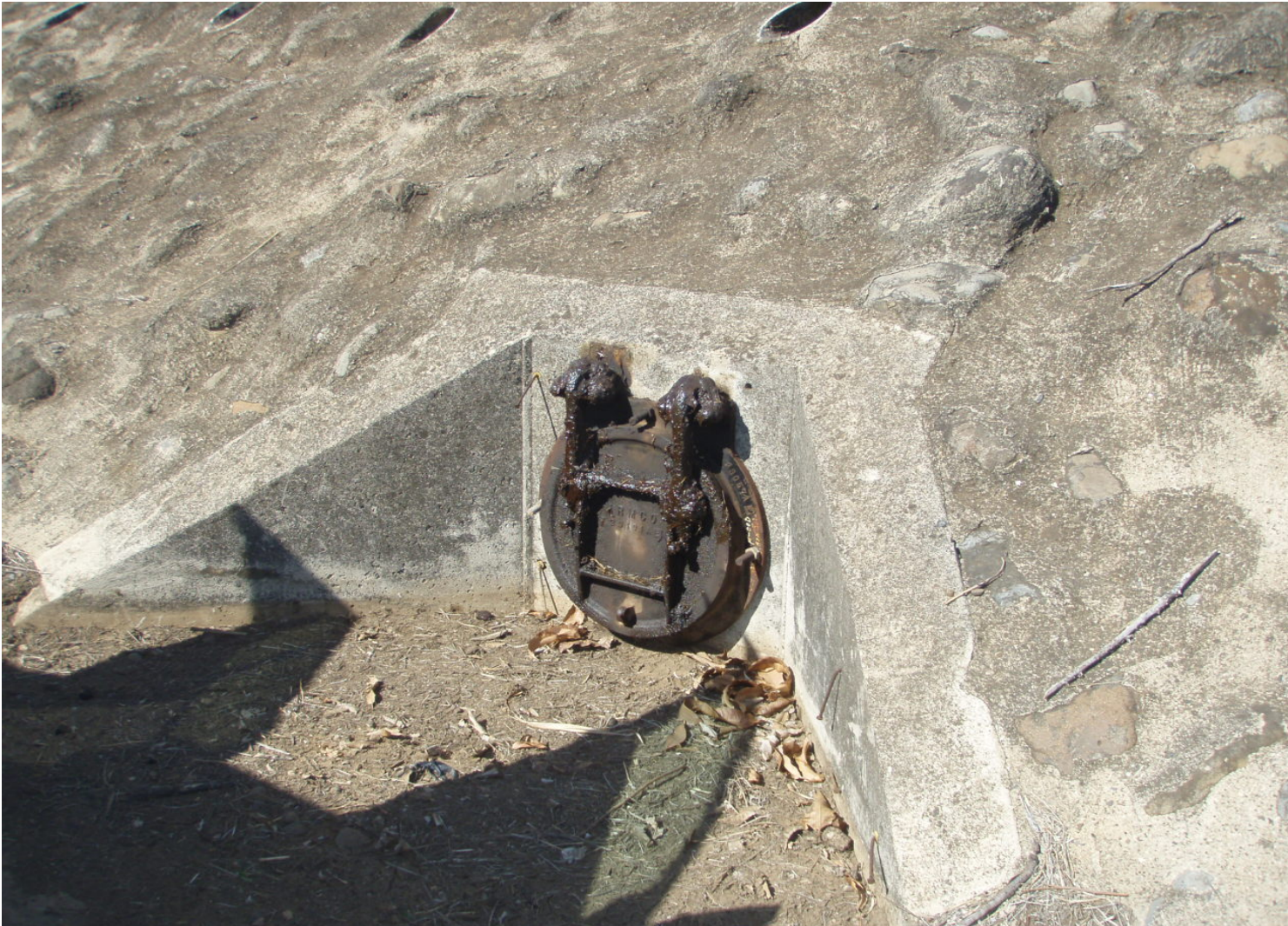
Inspect ID: ISLG_2009_a_0003 Name: Interior Drainage Caption: Sta.88+20, LB 24 inch flapgat in good condition & lubricated No debris or sediment build-up
