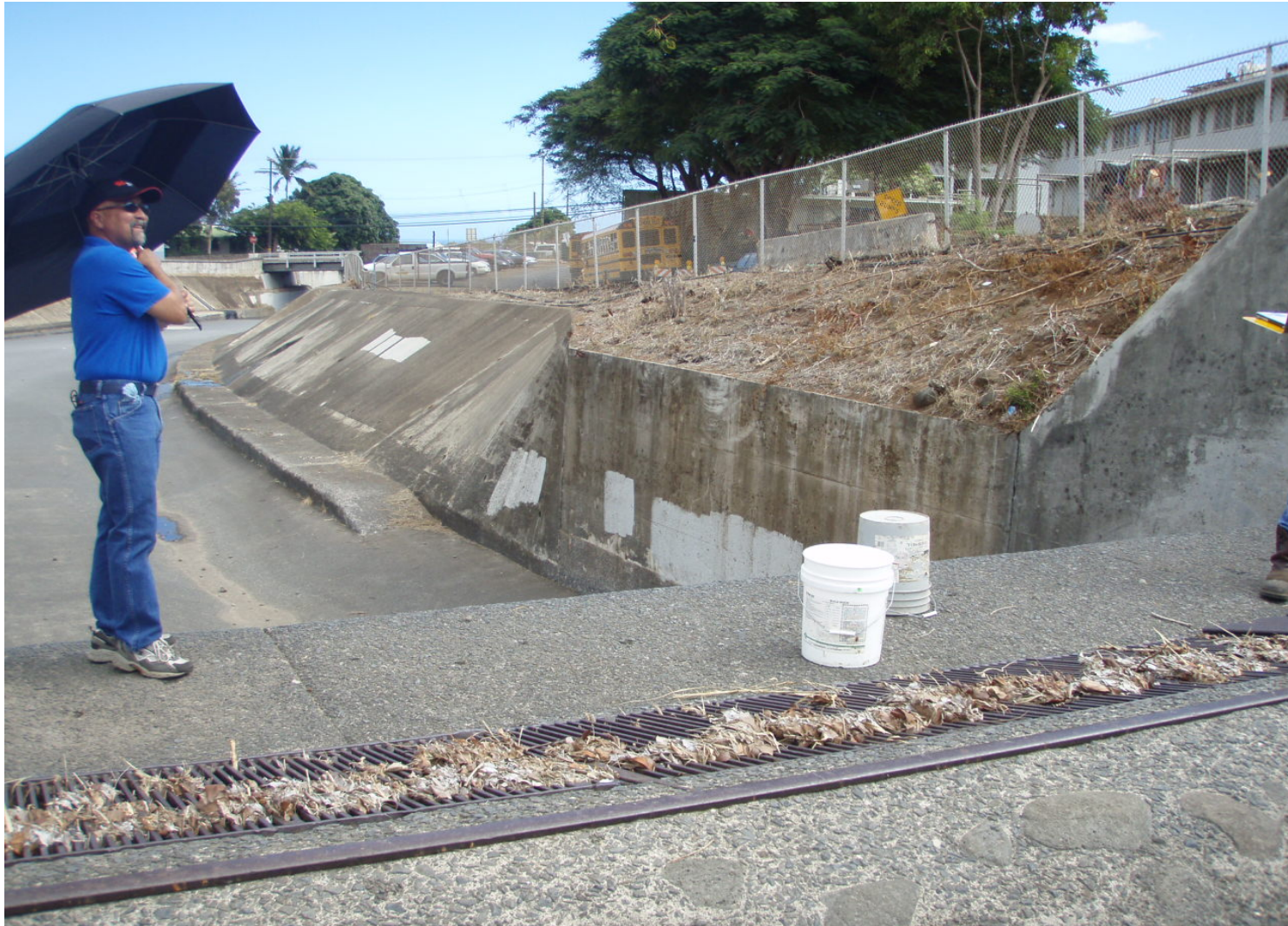
Inspect ID: ISHR_2009_a_0007 Name: Flood Reduction Channel Caption: Sta. 104+70, RB Drop structure # 4 ; HC&S Water intake
