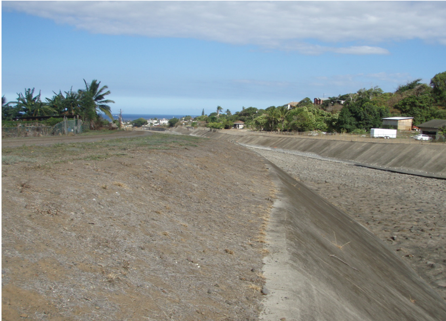
Inspect ID: ISHL_2009_a_0001 Name: Levee Embankment Caption: Sta. 125+50, LB, No vegetation on levee crown, no woody vegetation on sideslopes
