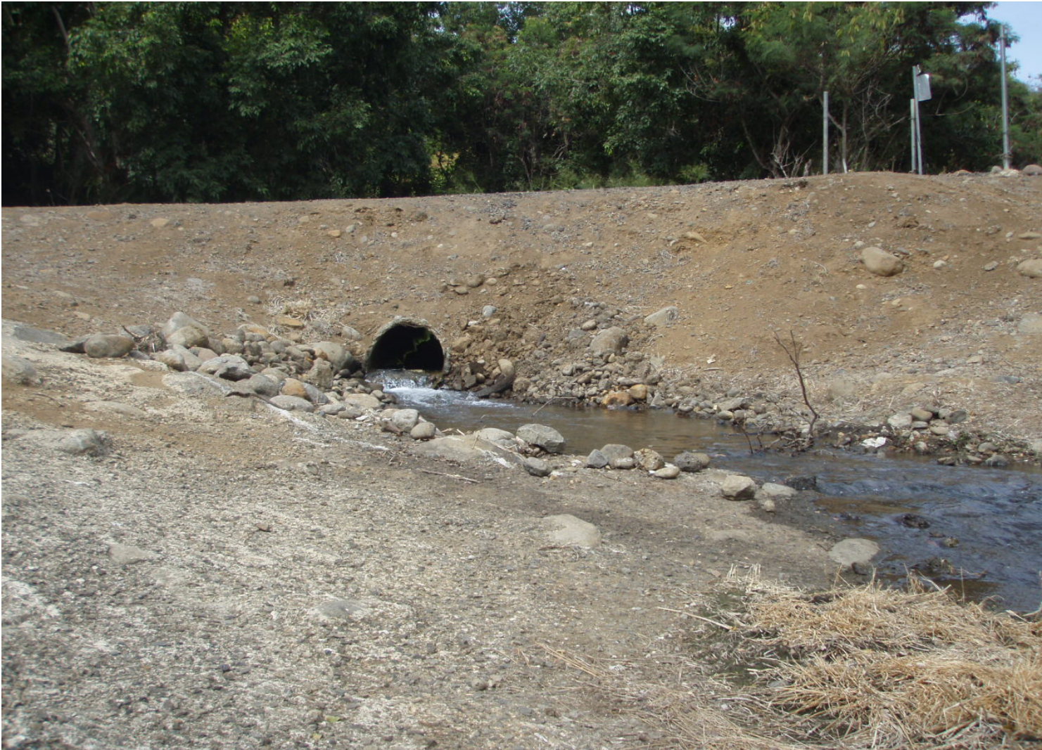
Inspect ID: ISIL_2009_a_0005 Name: Interior Drainage System Caption: Sta. 127+70, LB Culvert discharge pipe is in good condition no obstructions, continue to maintain.
