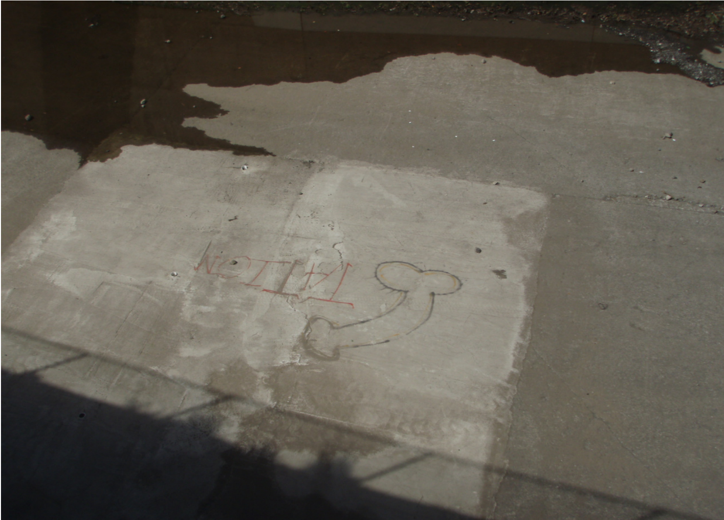
Inspect ID: ISHR_2009_a_0011 Name: Flood Reduction Channel Caption: Sta. 93+60, RB invert Concrete channel repaied at invert
