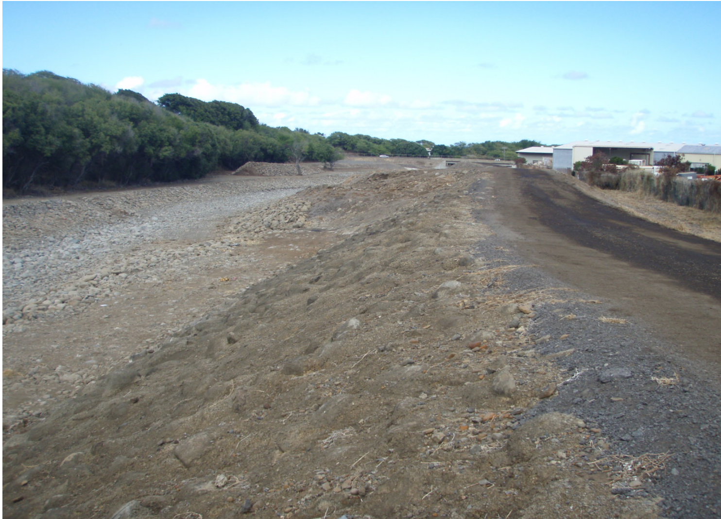
Inspect ID: ISLE_2009_a_0006 Name: Levee Embankment Caption: Sta. 33+10 (Levee A) Concrete slopelining in good condition
