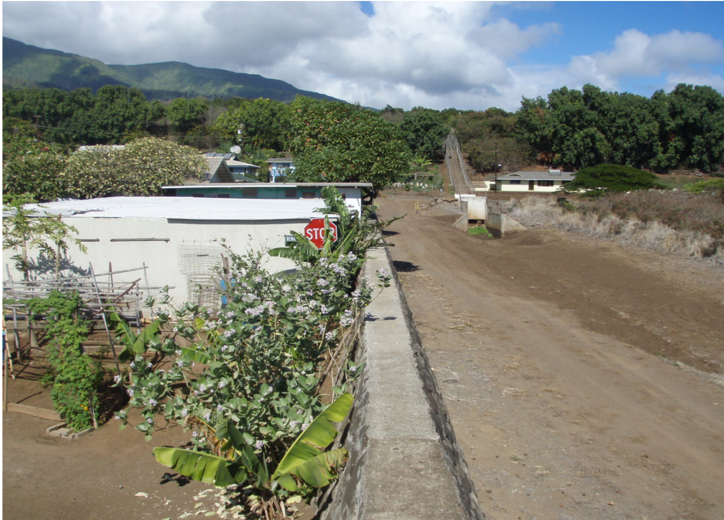
Inspect ID: ISLG_2009_a_0005 Name: Floodwall Caption: 24 inch flapgate in good condition floodwall in good contition Monitor
