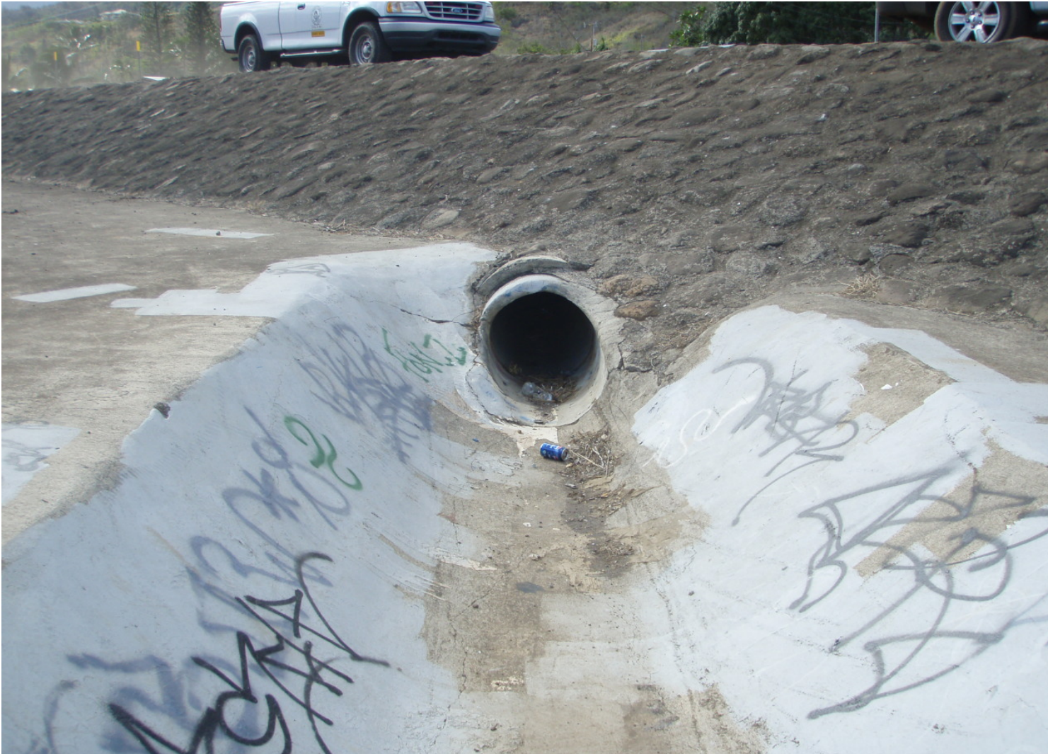
Inspect ID: ISHL_2009_a_0003 Name: Interior Drainage Caption: Sta. 113+40, LB No obstruction to concrete culvert, continue to maintain
