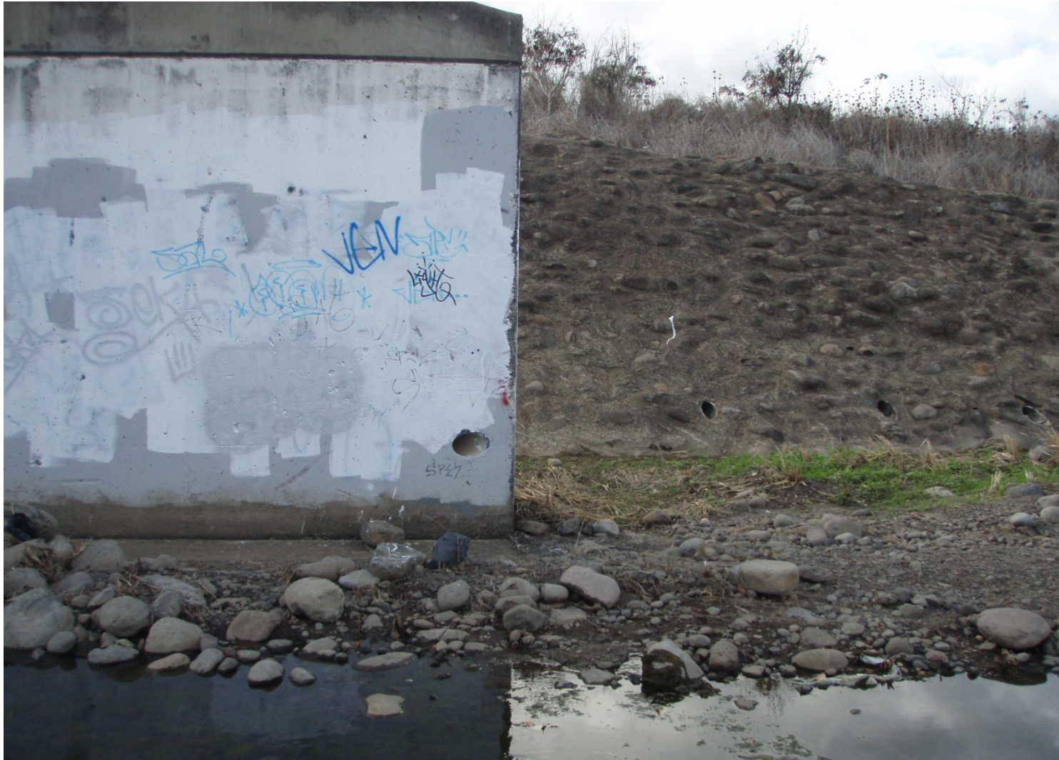
Inspect ID: ISHL_2009_a_0008 Name: Floodwall Caption: Sta. 92+40, LB Foundation ok, no scouring, low flow channel in good condition
