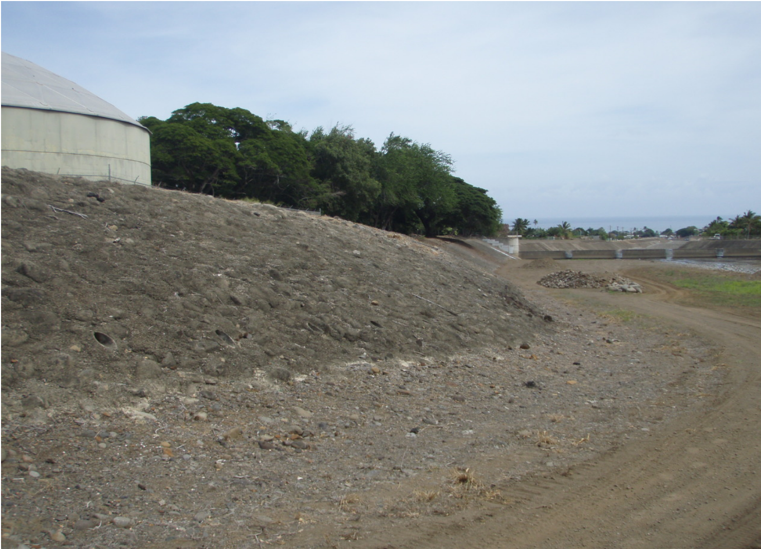
Inspect ID: ISIL_2009_a_0002 Name: Levee Embankment Caption: Sta. 136+20, LB, Typical condition of vegetation control, very good
