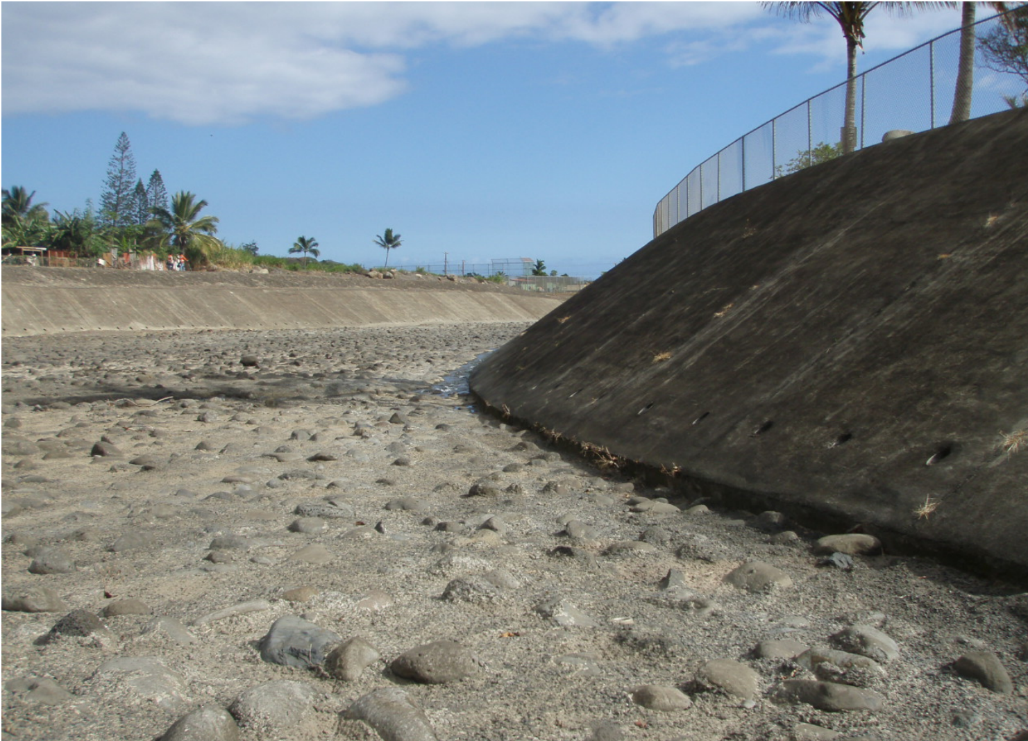
Inspect ID: ISHR_2009_a_0001 Name: Flood Reduction Chnl Caption: Sta. 125+90, RB No vegetation or debris in channel
