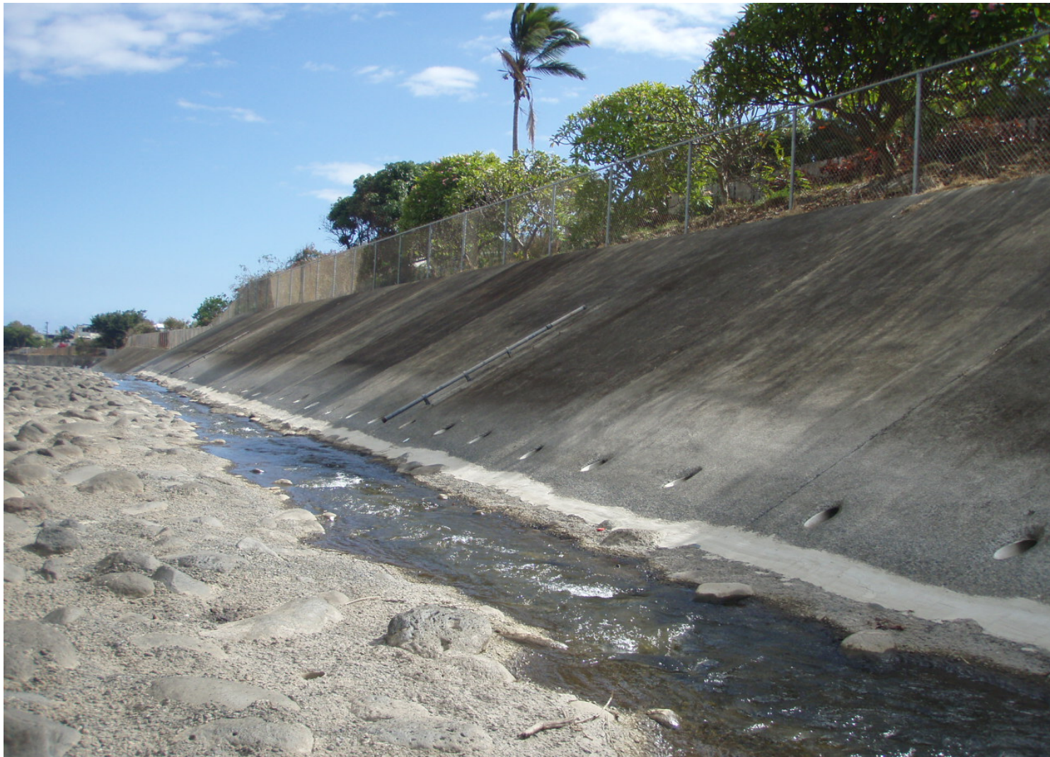
Inspect ID: ISHR_2009_a_0004 Name: Levee Embankment Caption: Sta. 116+30, RB Fencing replaced since previous inspection Concrete surface repaired at toe of sideslope
