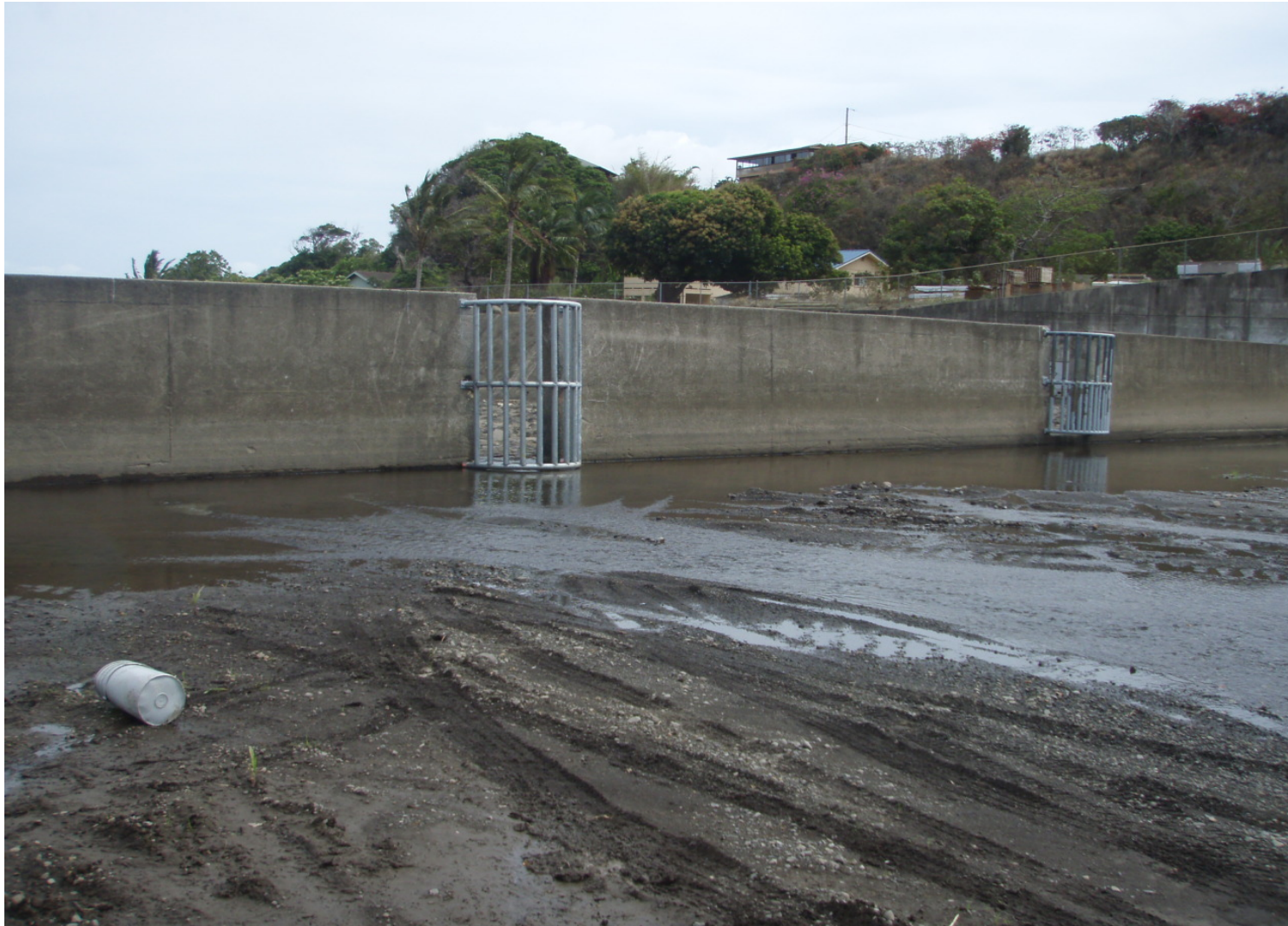
Inspect ID: ISIL_2009_a_0006 Name: Floodwall Caption: Sta. 127+60, LB to Centerline Gates have been repaired since last inspection. No rust, good maintenance.
