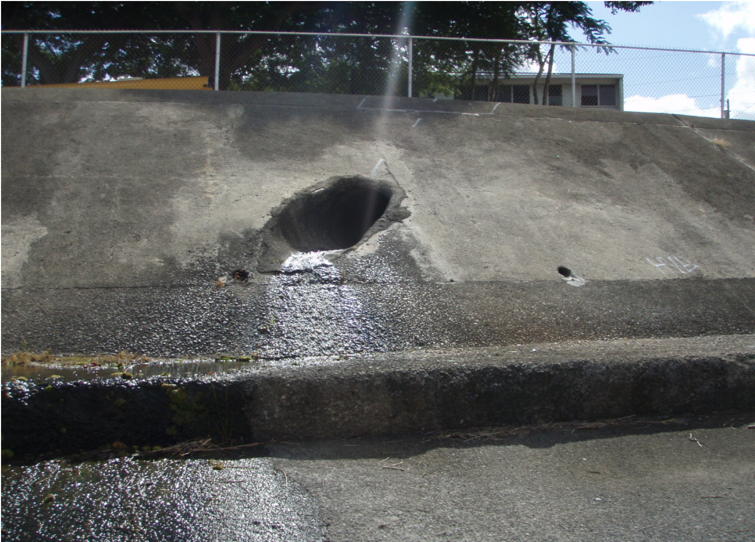
Inspect ID: ISHR_2009_a_0008 Name: Interior Drainage Caption: Sta. 103+30, RB 24 inch culvert in good condition, no obstruction adjacent to maintenance access ramp
