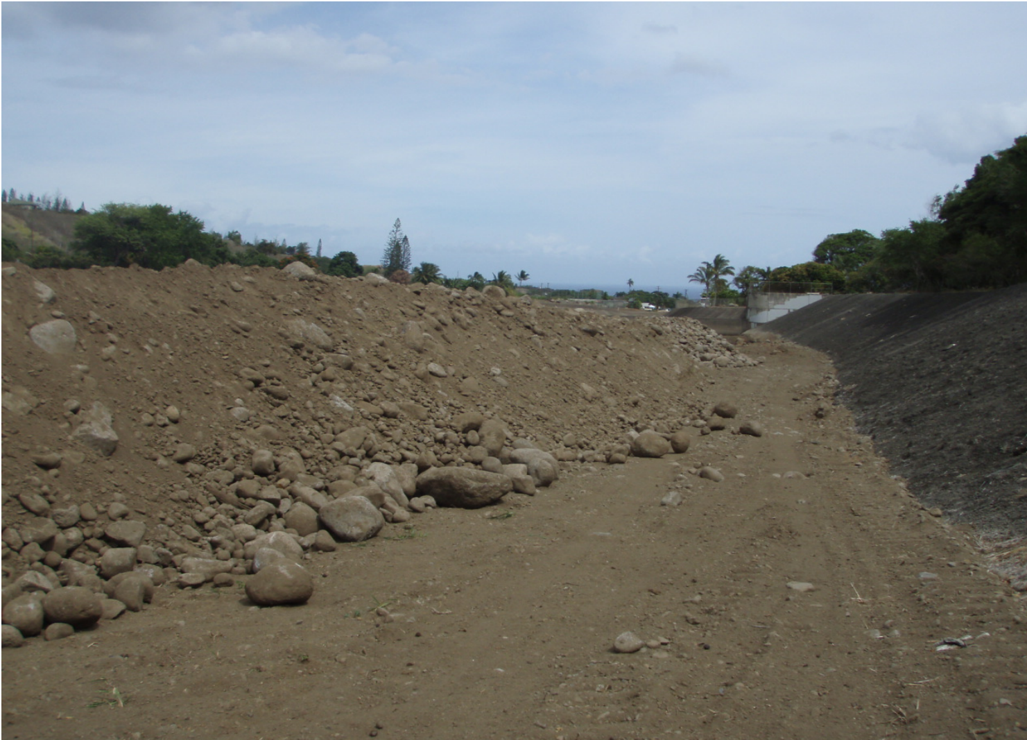
Inspect ID: ISIR_2009_a_0002 Name: Flood Reduction Chnl Caption: Sta. 133+50, RB Sholing minimally acceptable remove stockpile of sediments
