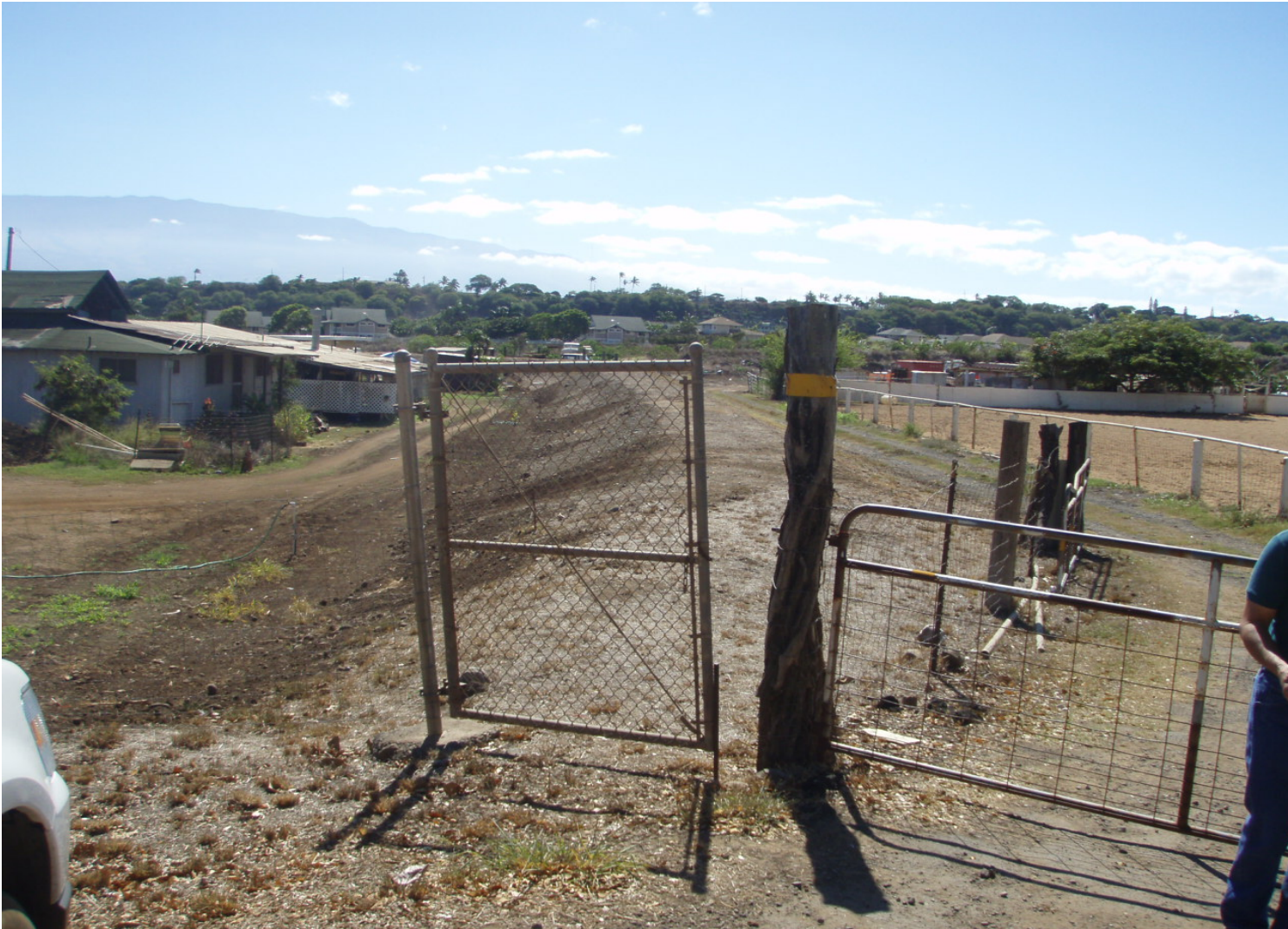
Inspect ID: ISLF_2009_a_0001 Name: Levee Embankment Caption: Sta. 51+50, LB Unwanted vegetation has been removed
