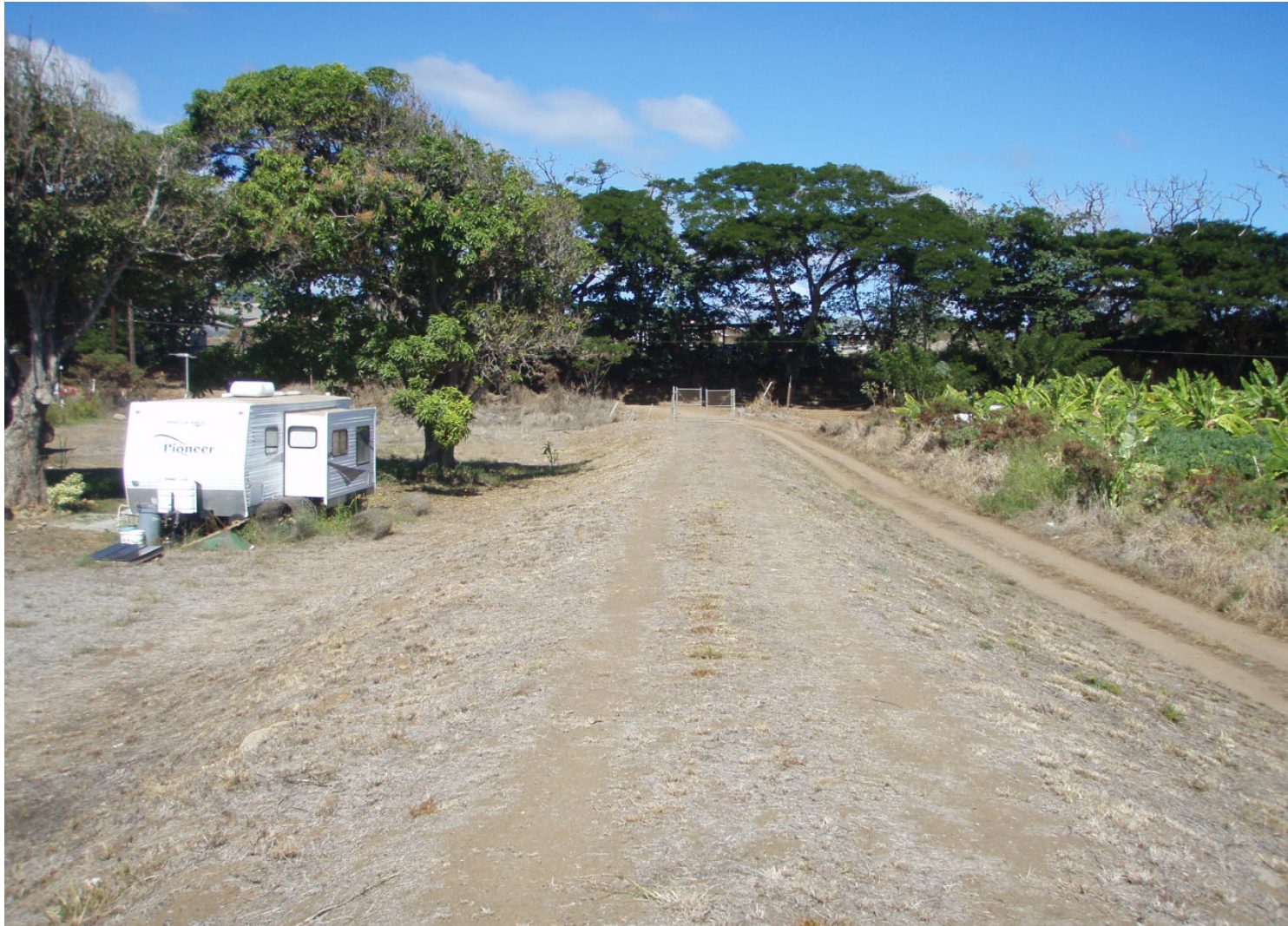
Inspect ID: ISLF_2009_a_0004 Name: Levee Embankment Caption: Sta. 51+20, LB 24 inch flapgate in good condition & lubricated Levee Crown and Sideslopes clear of all unwanted vegetation
