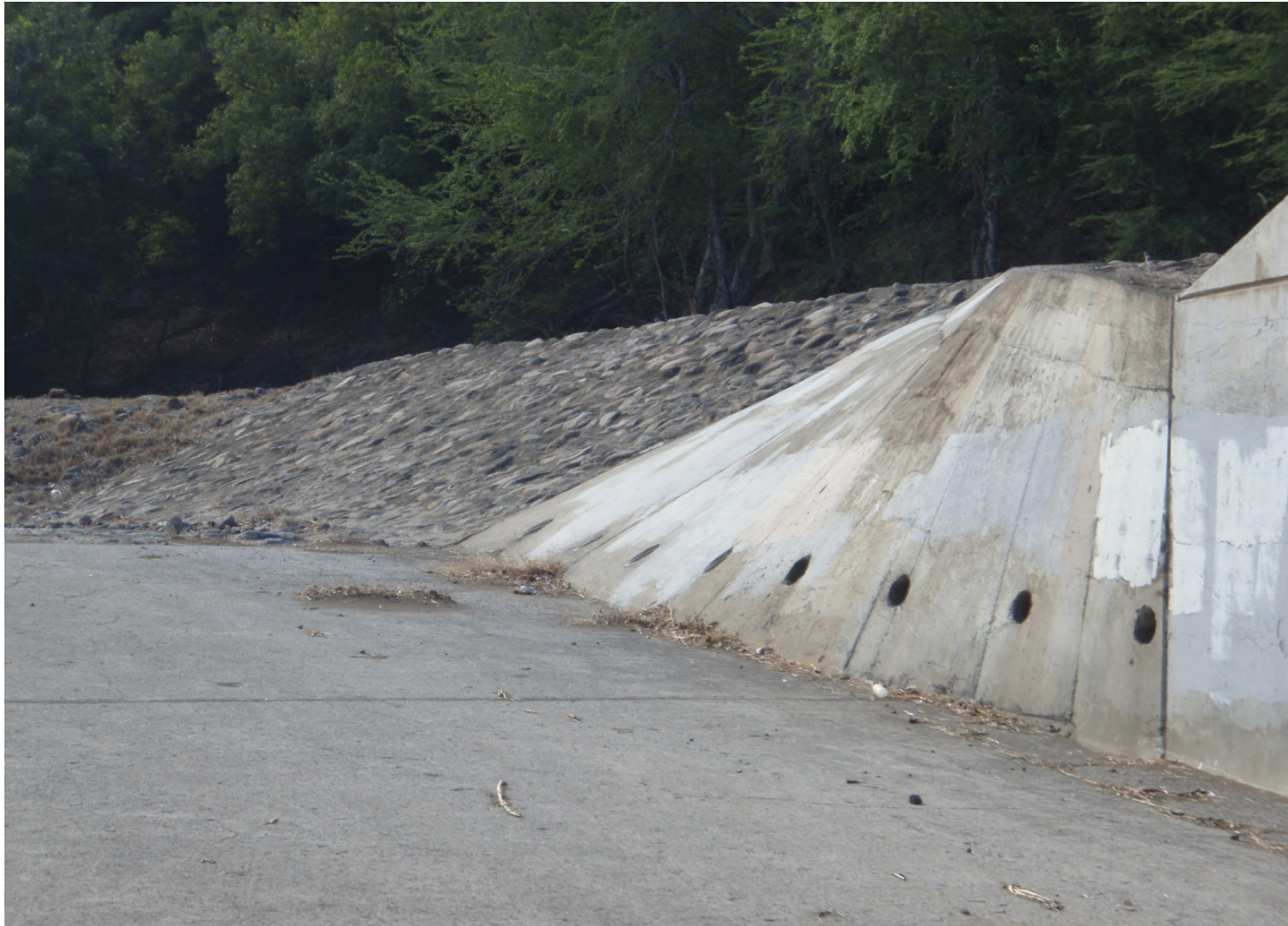
Inspect ID: ISAL_2009_a_0003 Name: Levee Embankment Caption: Sta. 22+00, LB Rippapbank protection in good condition
