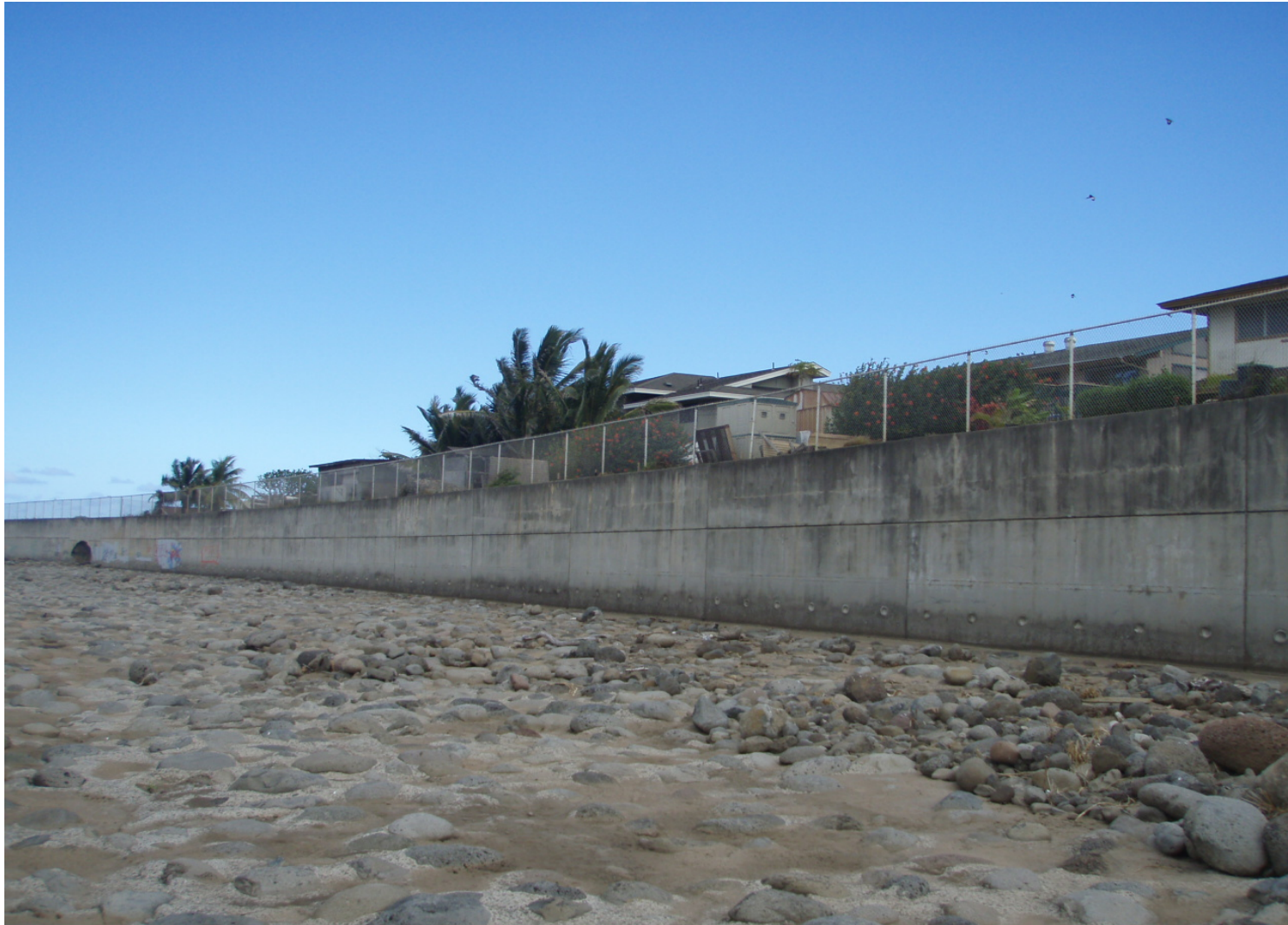
Inspect ID: ISAR_2009_a_0002 Name: Flood Reduction Channel Caption: Sta. 13+30, RB Approximately 7 properties have blocked the maintenance access way Unacceptable
