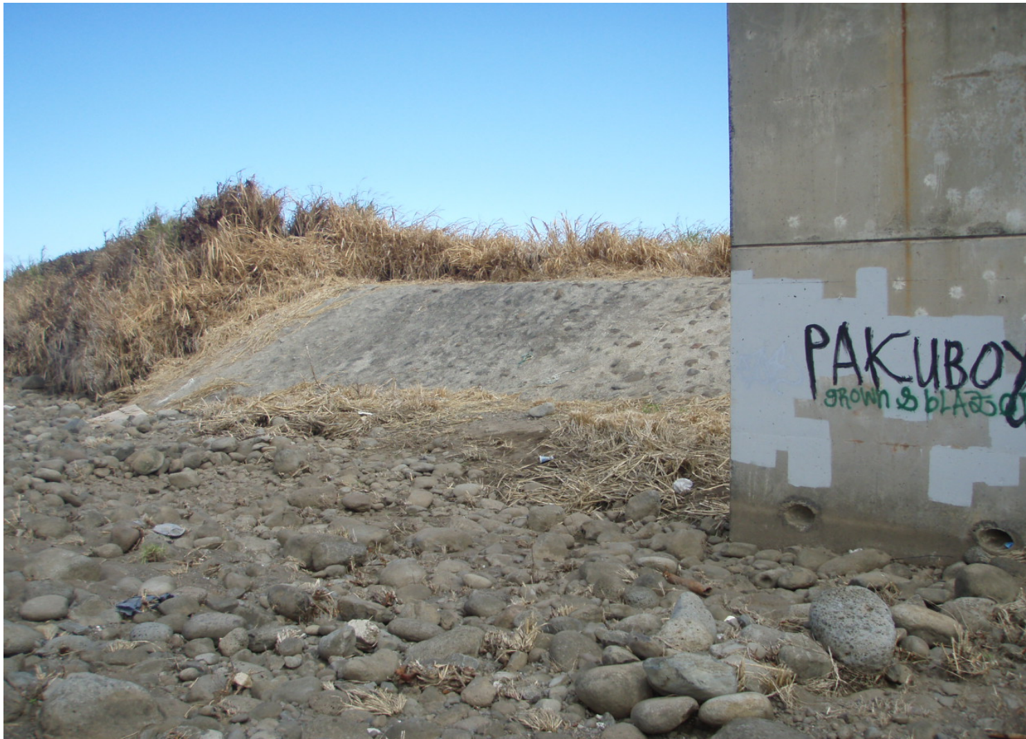
Inspect ID: ISAR_2009_a_0004 Name: Levee Embankment Caption: Sta. 5+40, RB End of flood control channel, riprap bank protection in good condition Fence in good repair
