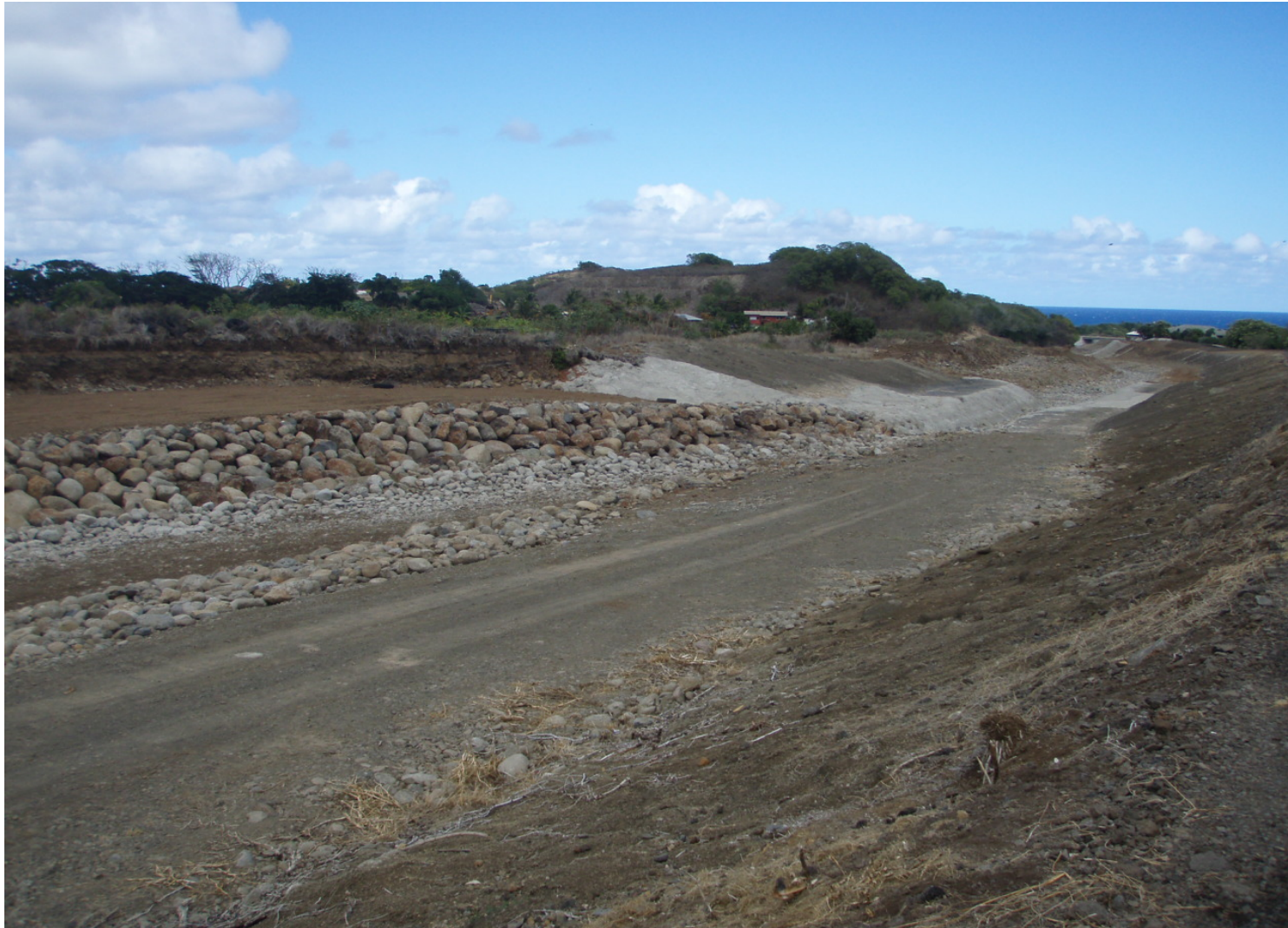
Inspect ID: ISLE_2009_a_0004 Name: Levee Embankment Caption: Sta. 51+10 (Levee C) Repairs have been made to stabilize the levee
