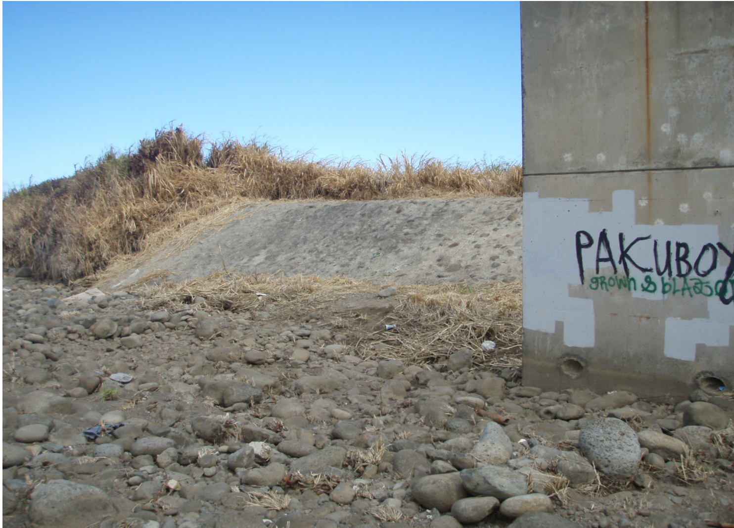
Inspect ID: ISAR_2009_a_0004 Name: Levee Embankment Caption: Sta. 5+40, RB End of flood control channel, riprap bank protection in good condition Fence in good repair
