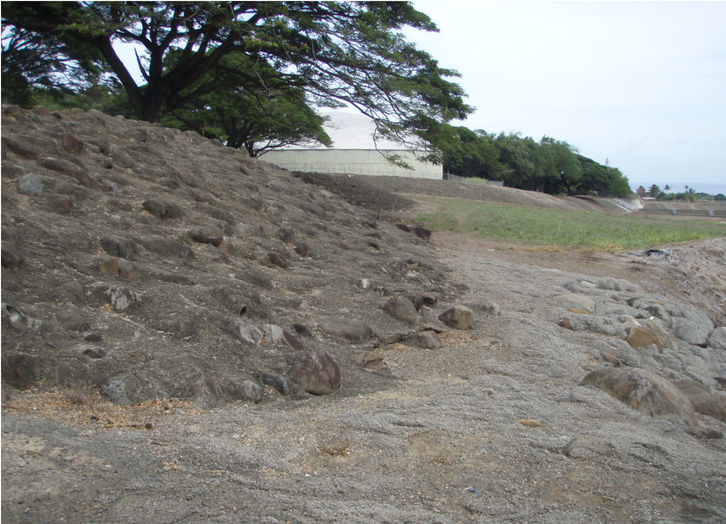
Inspect ID: ISIL_2009_a_0001 Name: Levee E Caption: Sta. 139+20, LB, P-1 No woody vegetation on sideslope or crown, good maintenance
