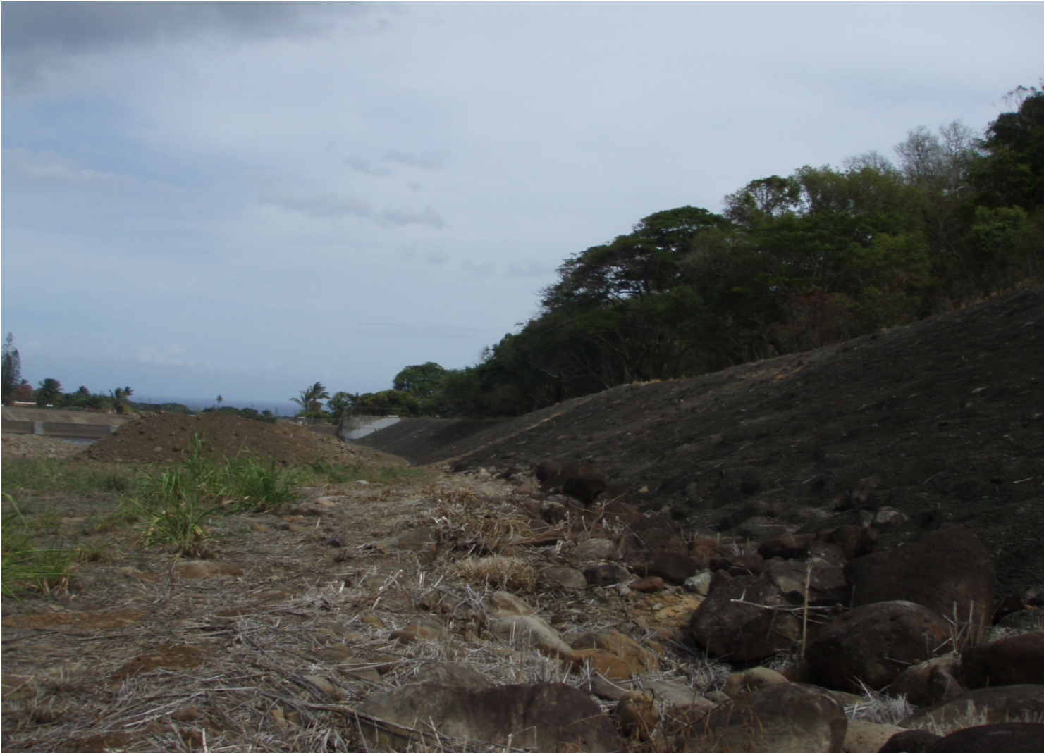
Inspect ID: ISIR_2009_a_0001 Name: Levee Embankment Caption: Sta. 134+80, RB No woody vegetation, weep holes clear.
