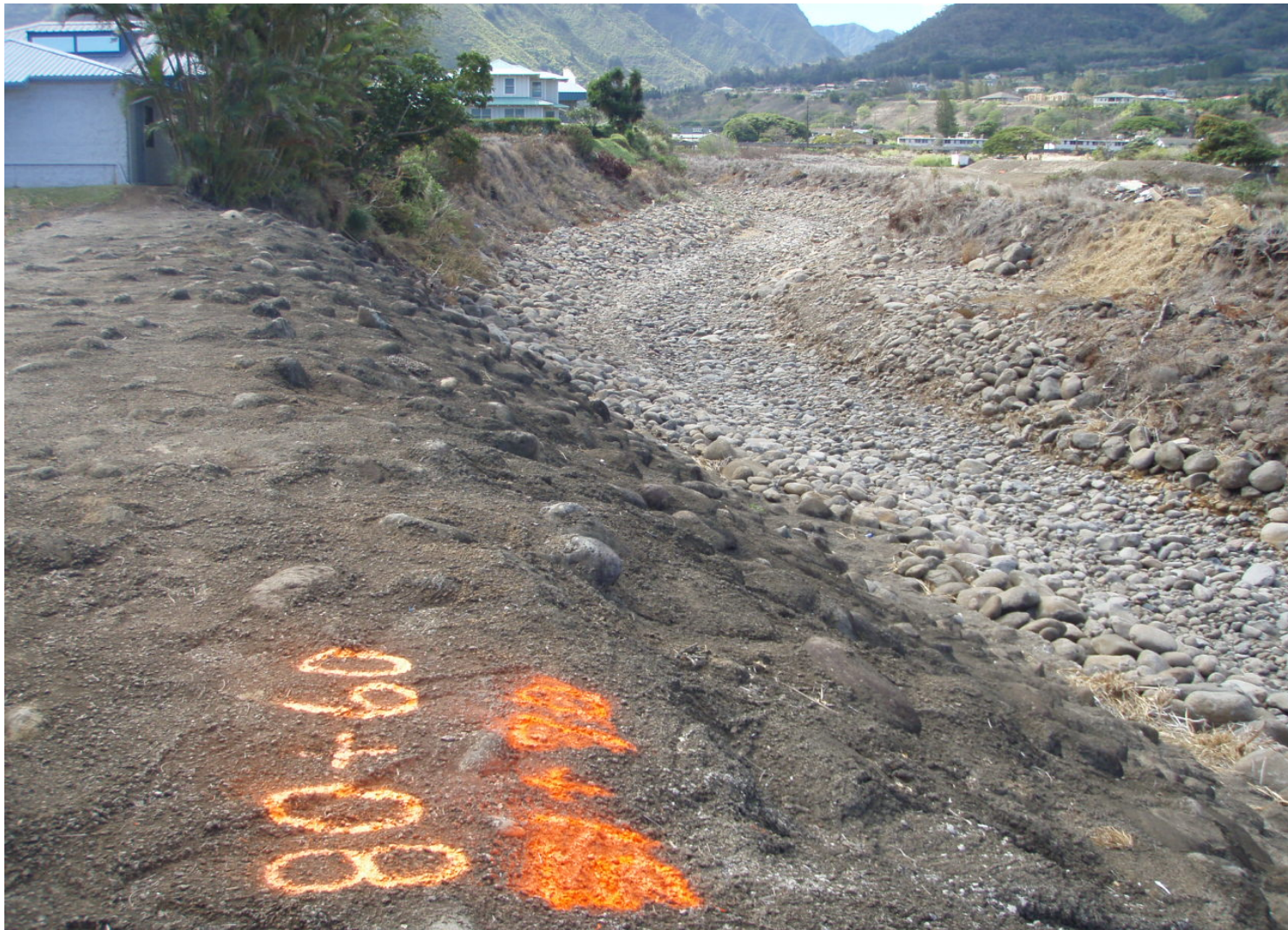
Inspect ID: ISLE_2009_a_0002 Name: Levee Embankment Caption: Sta. 80+60, (Levee E) Vegetation removed, chnl cleaned
