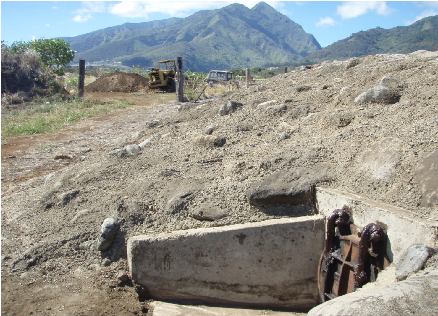
Inspect ID: ISLF_2009_a_0003 Name: Interior Drainage Caption: Sta. 51+30, LB 24 inch flapgate in good condition and lubricated Encroachment //// Verify easement at toe of levee //// Fence
