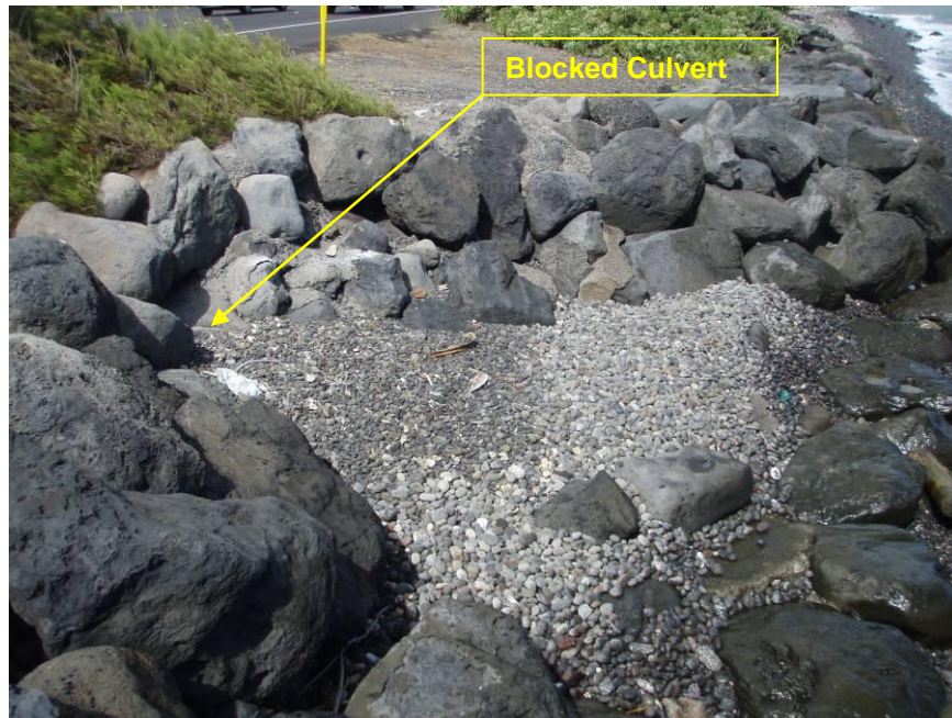
h. Sta. 7+81, Monitor void at the crest. Road culvert blocked.
