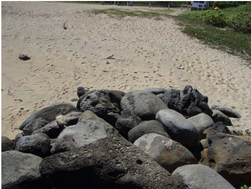
o. Sta. 16+00, Monitor sand erosion at tie-back.
