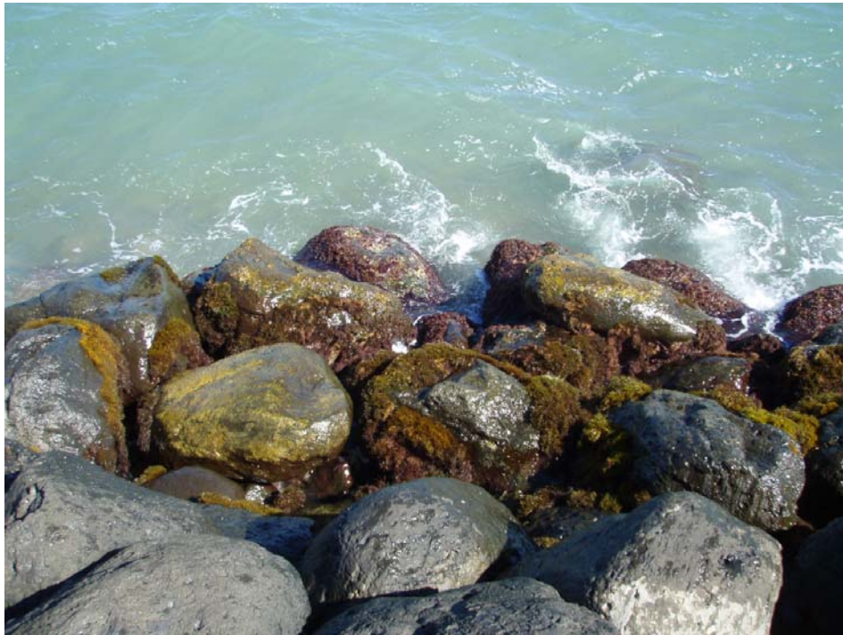
d. Sta. 12+50, Monitor void and bridging armor stone on the sideslope. minor change this year.
