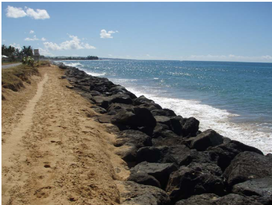
f. Sta.14+90, 1 Perched armor stone with void, monitor this area.
