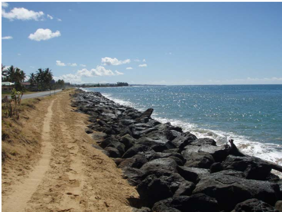
h. Sta. 16+70, 1 flipped armor stone, monitor this area.
