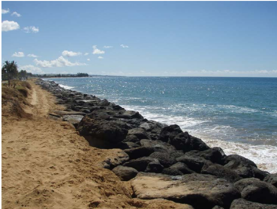
g. Sta. 15+38, Overview, perched armor stone, monitor this area.
