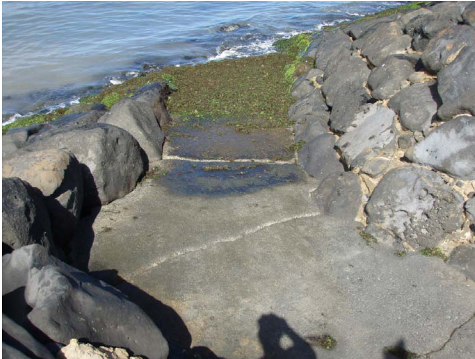
j. Sta. 8+73, 2 nd , access walkway, repair cracks in sidewalk as needed.
