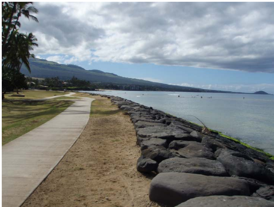
q. Sta. 23+00 to Sta. 20+00, Overview, backfill eroded area filled sidewalk new this inspection.
