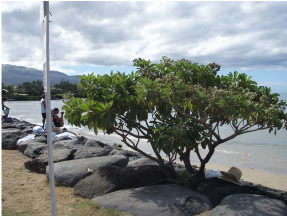
t. Sta. 24+50, Remove tree from revetment.
