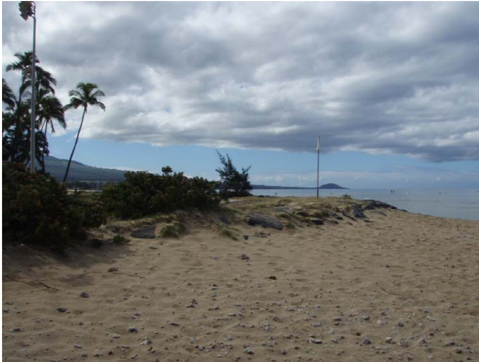
p. Sta. 13+80, No Change since FY04. Remove the vegetation from revetment .
