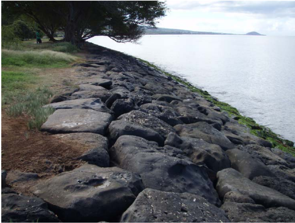
f. Sta. 3+76, to Sta. 4+06, Monitor the area adjacent to cracked armor stone for settling.
