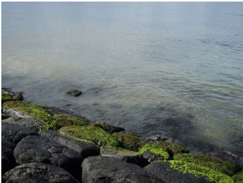
g. Sta. 3+96, 1 ea. Displaced armor stone, void at toe. Monitor Sideslope.
