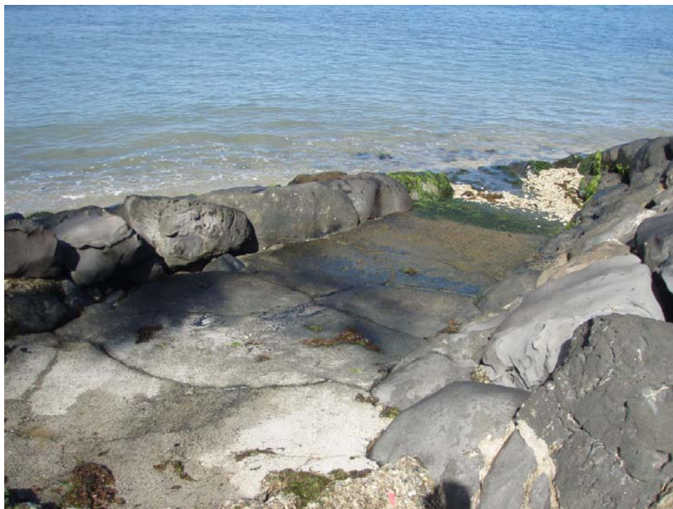
c. Sta. 3+00, 1 st access walkway, repair cracks in sidewalk as needed.
