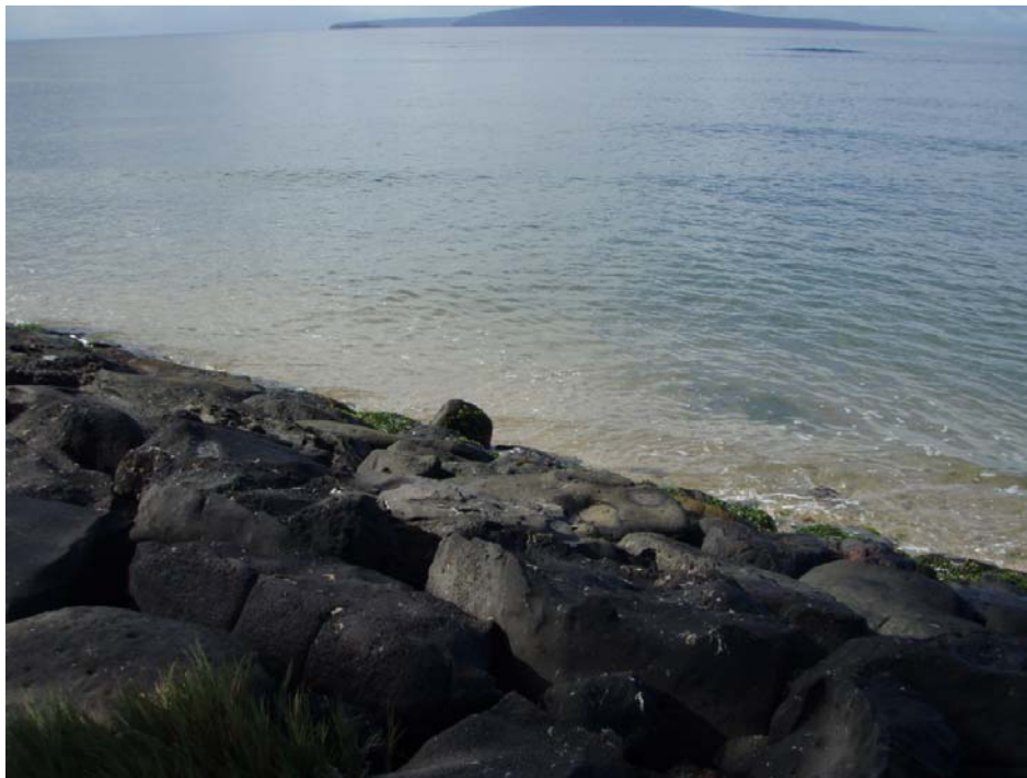
e. Sta. 3+48, Monitor the armor stone resting adjacent the toe. Minor change this year. No obvious voids.
