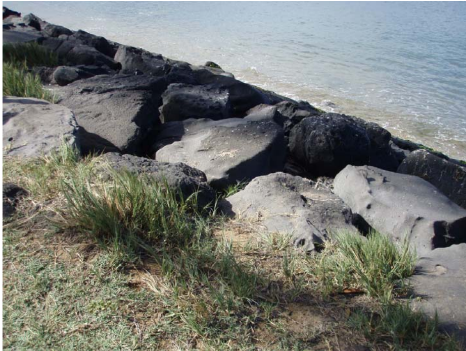
d. Sta. 3+20, Monitor minor settling at hinge. No Change.
