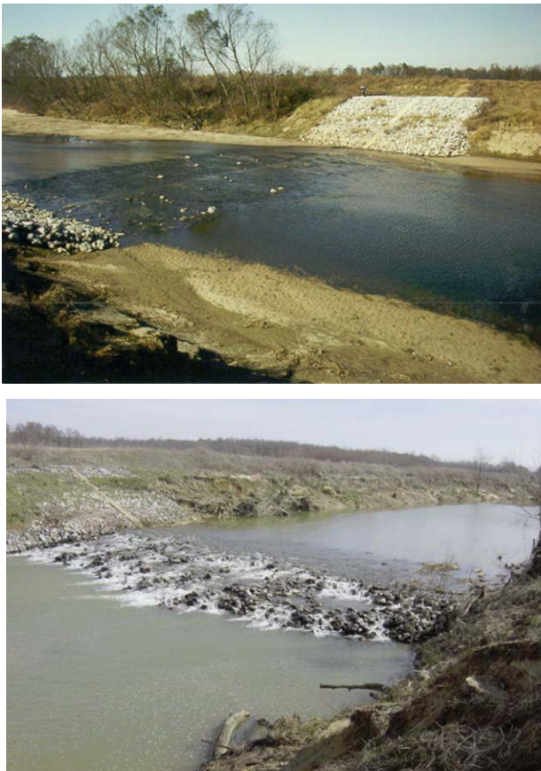
Figure 4. Riprap sills post-construction (above) and during 2003 inspection (below). From Biedenharn et. al, 2004.
